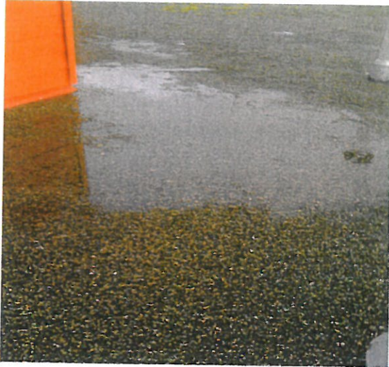
Roof adjoining old hose tower, more ponding, weight, ponding at seem of structure.
