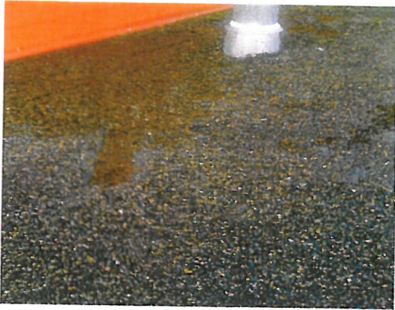
Pondling at old hose tower structure front side at roof.
