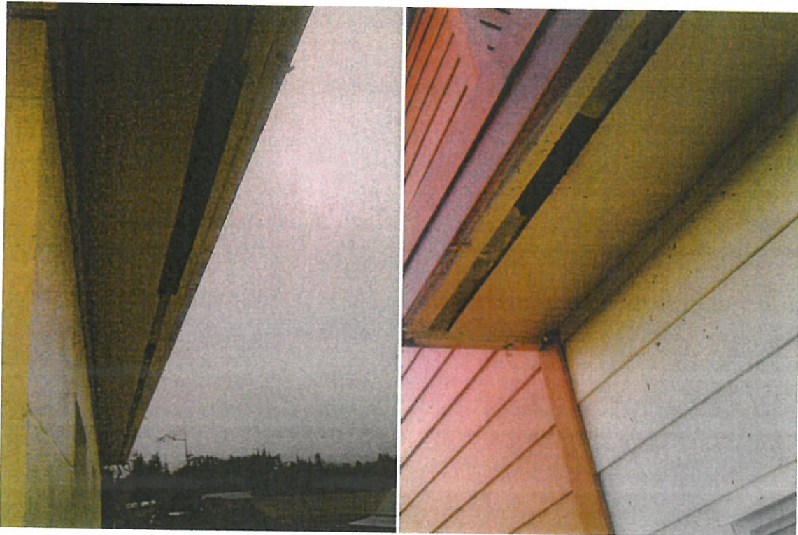
Roof venting, there are many fixes here with different types of methods, due to age, birds are making egress easily for nesting, etc..
