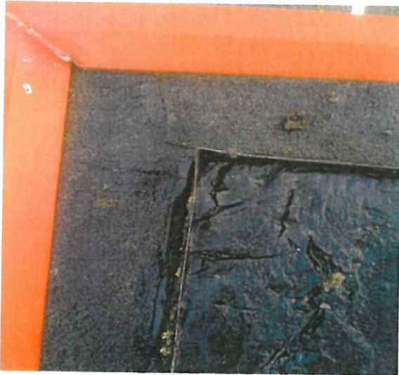
Exposed tar, no gravel to protect, cracks which make good egress of water to interior.
