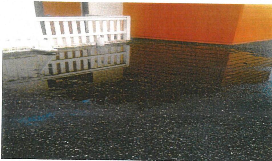
The pooling you see here is called "pondling", location here is outside the upper training room classroom. One of the issues here is the added weight of water on our structure, also improper location of drains.
