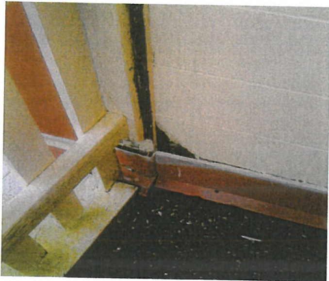
Location upper training room door, part of cinderblock is missing, and flashing not adhere to building.
