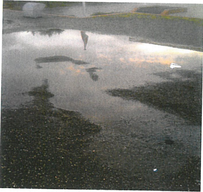
From the last photo, turning 90 degrees, facing flag pole, more pondling, added weight and improper drainage.
