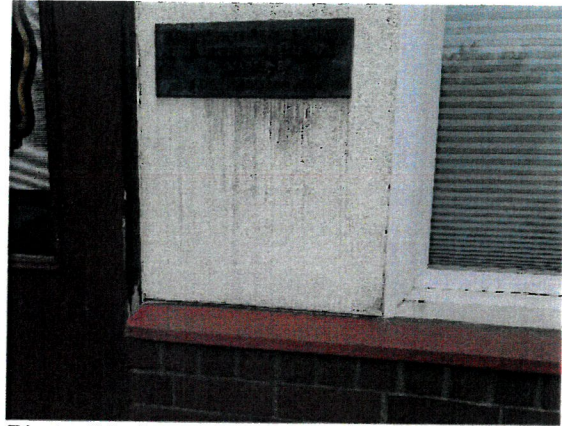
Photo 26: Stucco – Exterior Front (ND)
