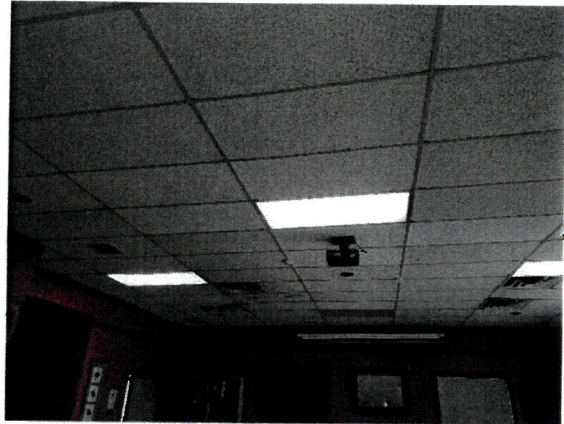
Fluorescent Light Ballast; Fluorescent Tube Lights (PCB; Mercury)
