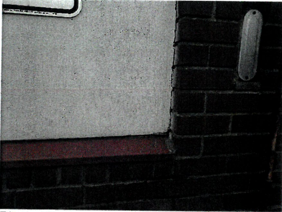
Photo 25: Stucco – Exterior Front (ND)
