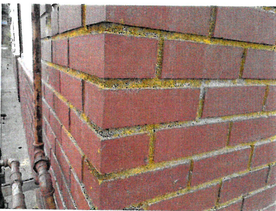
Photo 29: Mortar – Exterior Front (ND)
